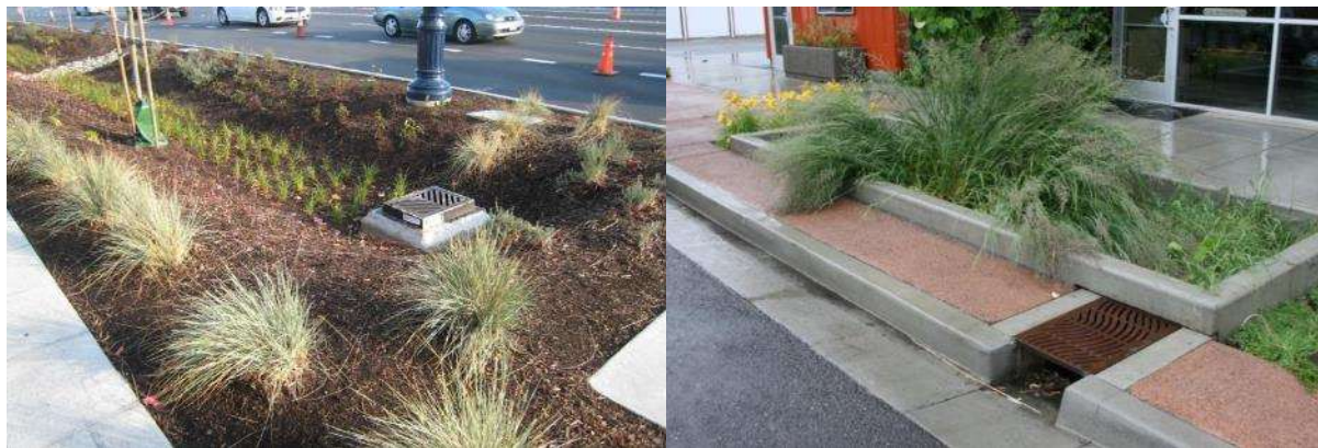
Figure 5-7: Offline conveyance system (left) versus Online conveyance system (right). (Montana Department of Environmental Quality, 2017)
